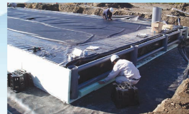
▲ Medium-sized underground water storage tank under construction: with a water storage capacity of 95 m 3 .
