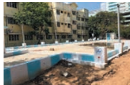
6 The upper area is ready to be used as a parking lot
